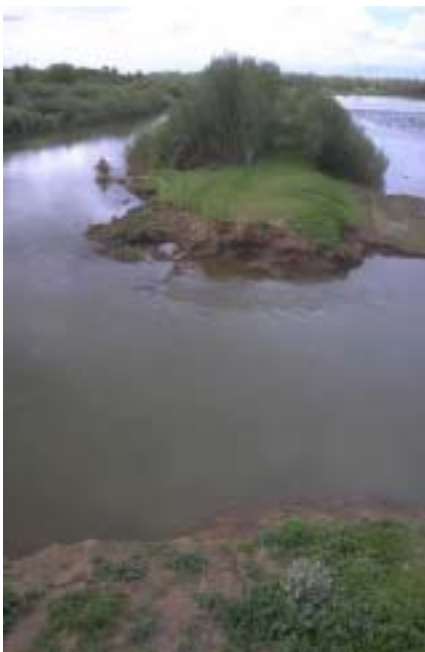
CLOSEUP OF THE LEVEE BREACH
